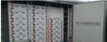
Nova Scotia, CAN x2 1.12MWh / 500kW
