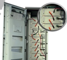
Ontario, CAN 502kWh / 150kW
