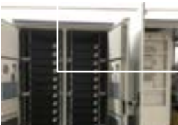
Ontario, CAN 100kW/368kWh (HW+SW)
