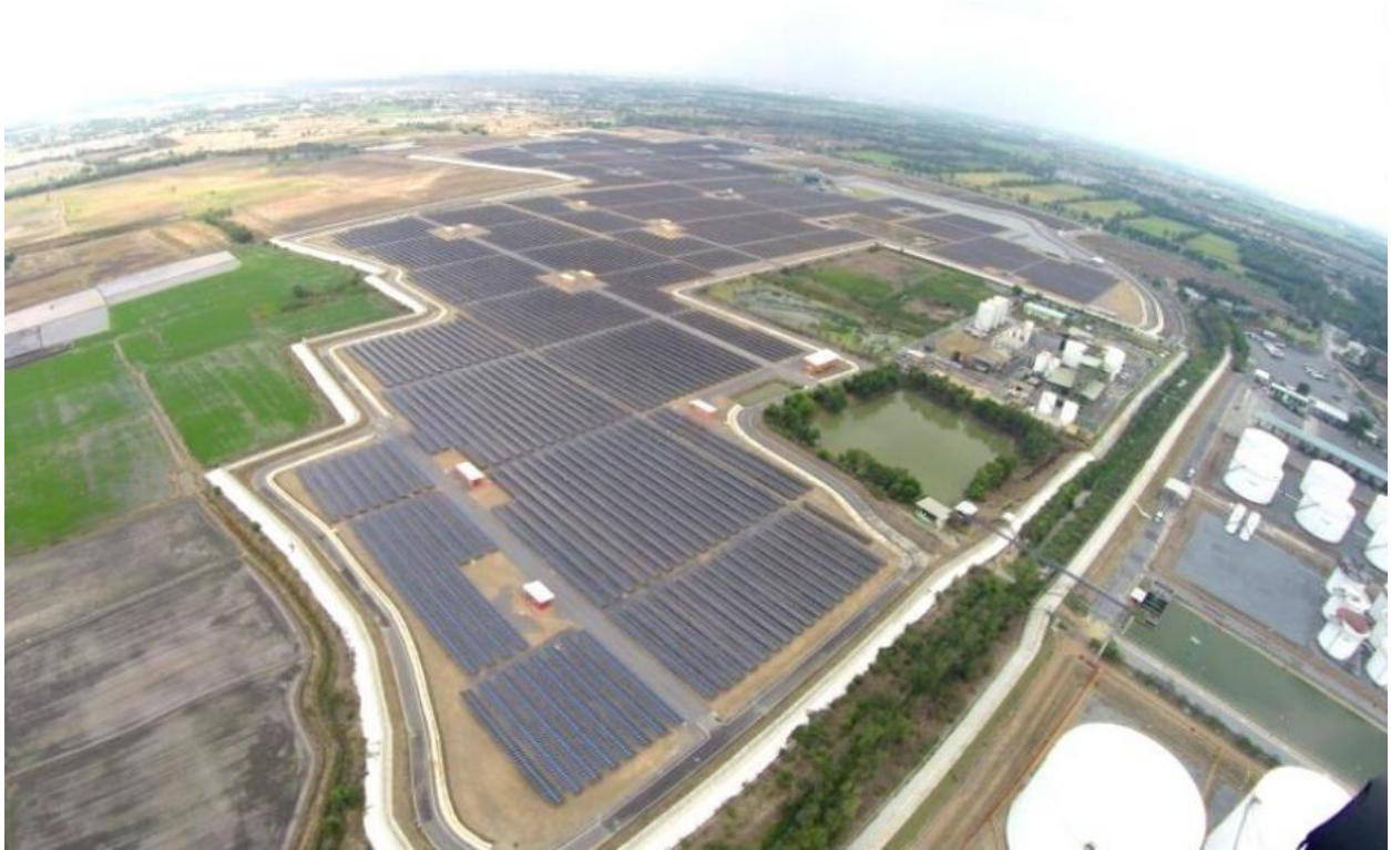
Bang Pa in solar farm, 44MW with NanoPV group system design and Engineering, 2014.
