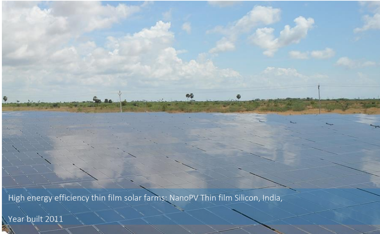
Solar Farm with capacity of 1.563MW, Built in 2010
