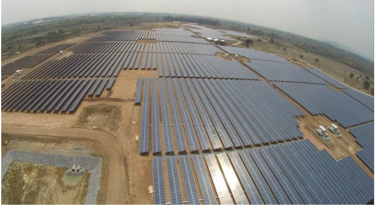
Bum net narong solar farm, 25MW capacity with NanoPV system design and Engineering 2013.
