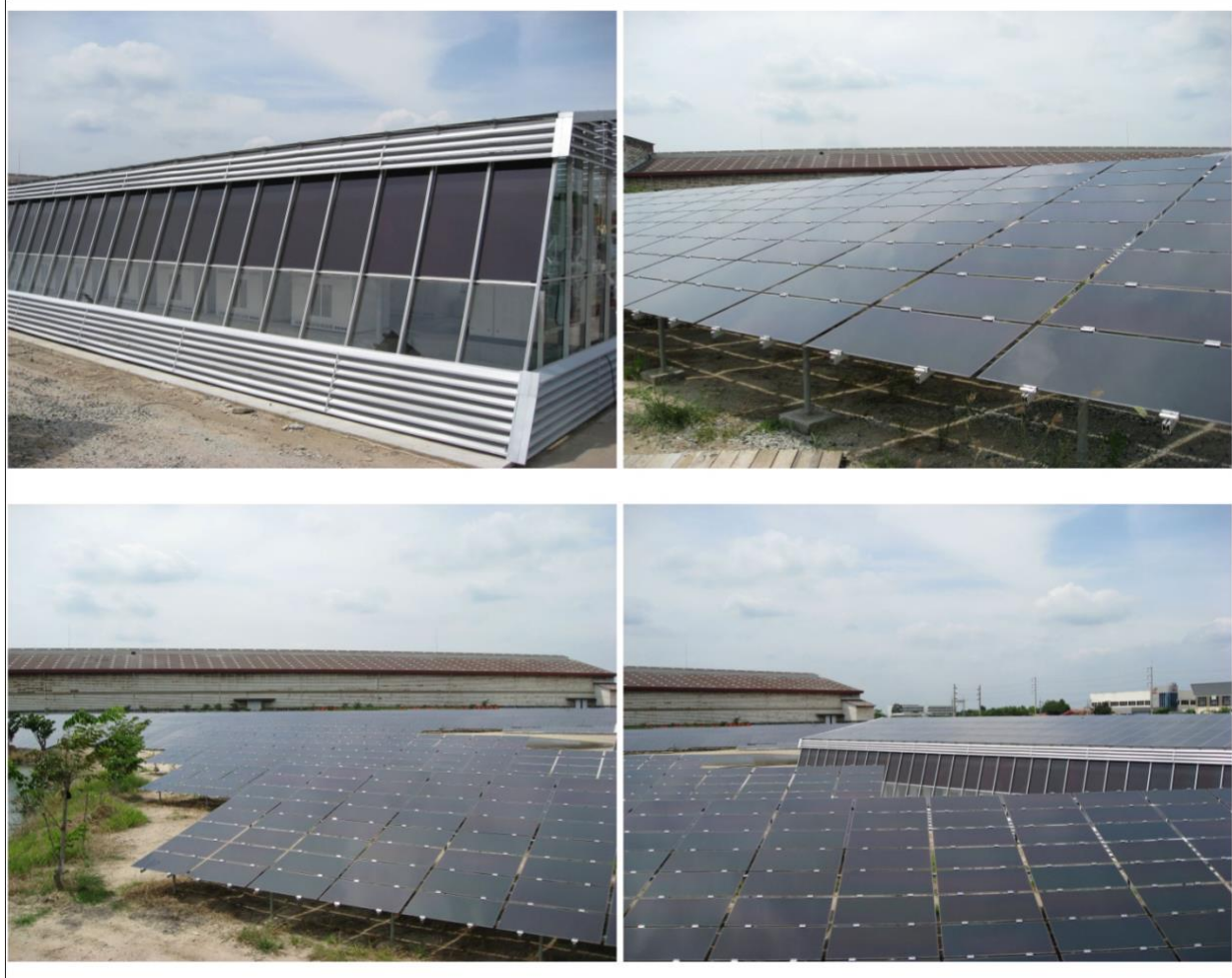
Power plant using NanoPV Thin film technologies. Built in 2007
